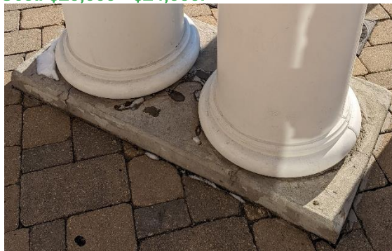
Cracked concrete at column bases.
